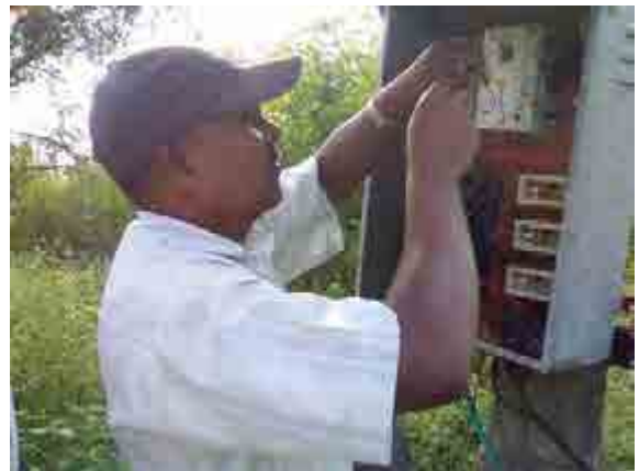
Figure 51: A local village electrician is vital for ICT implementation in irrigation
